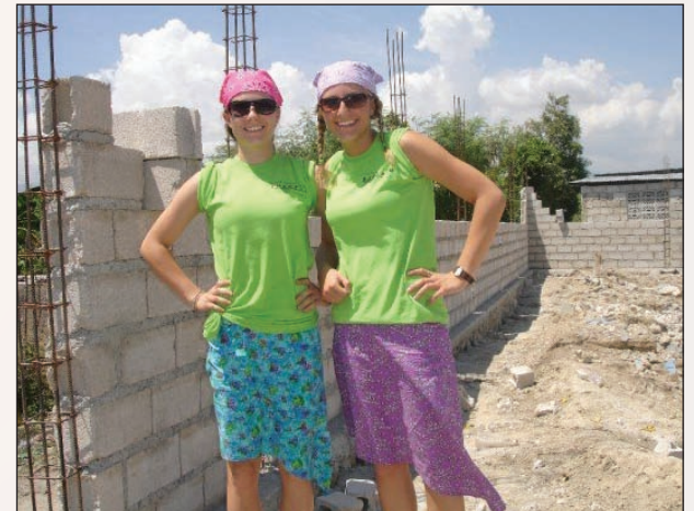
Sisters Brooke (left) and Mallery Thurlow (right) on the site of a school they built in Haiti.
